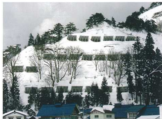
斜面下の集落を雪崩から守る (福島県耶麻郡西会津町) Snow-supporting structures which protect villages. (Nishiaizu Town, Maya Gun, Fukushima Pref.)
