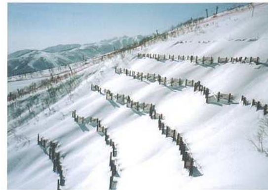
雪崩予防柵 雪崩発生区に設置し、雪崩の発生を未然に防ぎます。(長野県北安曇郡白馬村) Avalanche-prevention Fences Fences are installed in avalanche start zones. (Hakuba Village, Nagano Pref.)
